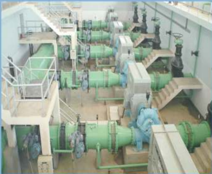
Kirloskar Butterfly, Sluice and Dual Plate Check Valves installed at Saurashtra pipeline Project, Gujarat, India
